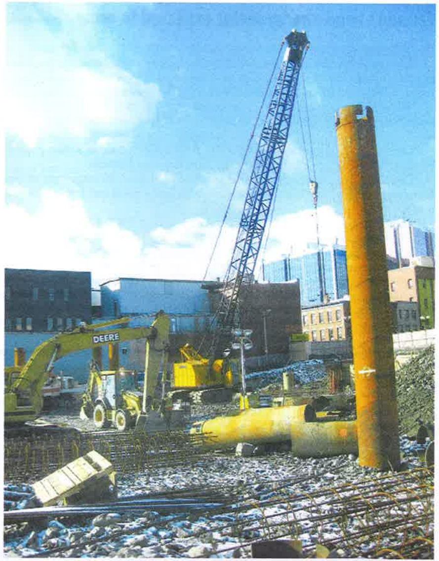
Crews use a 60-ton Link-Belt LS128 crawler crane to hoist casing and install rebar cages and concrete caissons for the seawater heating and cooling system of a 12-storey office building in St. John's, Nfld. Photo by Saul Chernos
